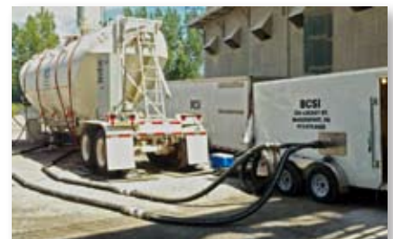
Sorbent supply is mixed and metered during trial burns for mitigation of emissions gases, metals and Hg.
